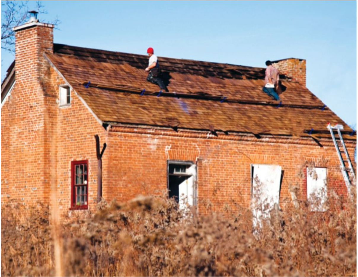
Folk Studies graduate assistant James Miller and undergraduate folklore minor Kohl Threlkeld replacing the roof of the Gardner House.
