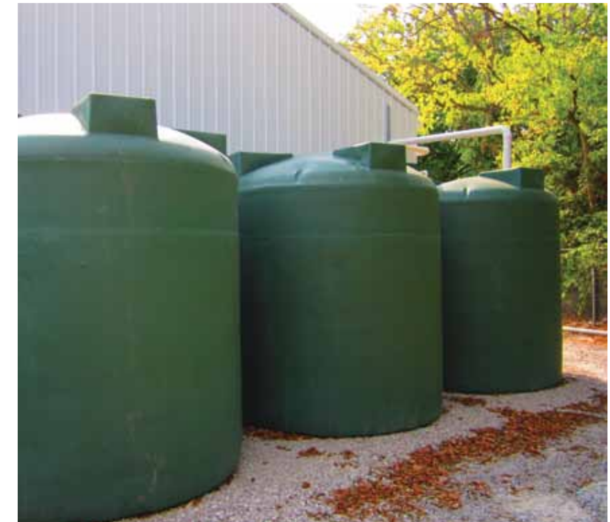
Collection System at South Street
