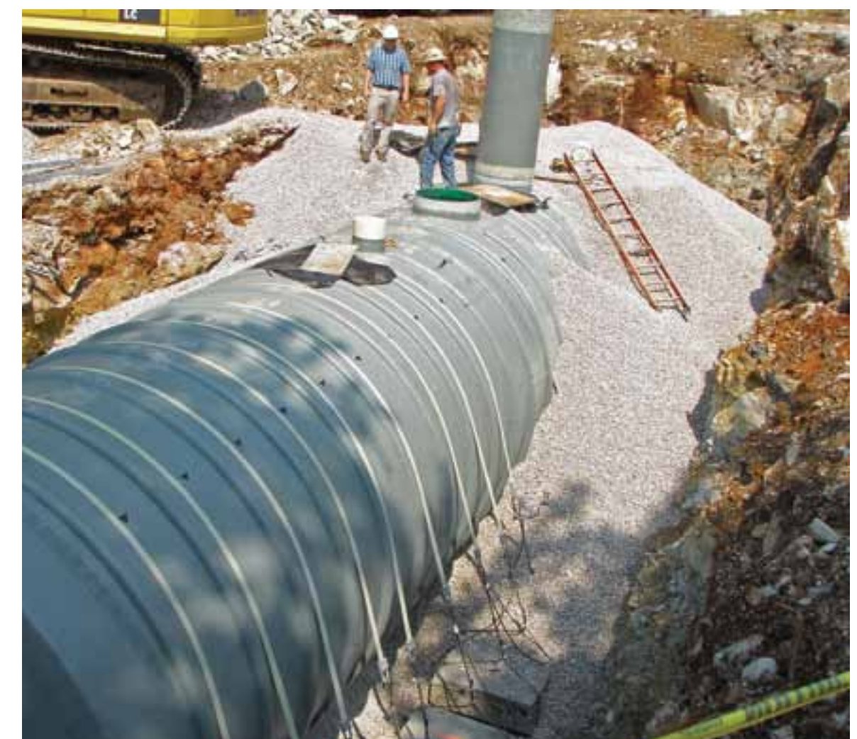
Subsurface collection cistern at Music Hall
