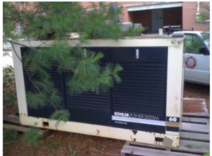
Kohler natural gas generator
