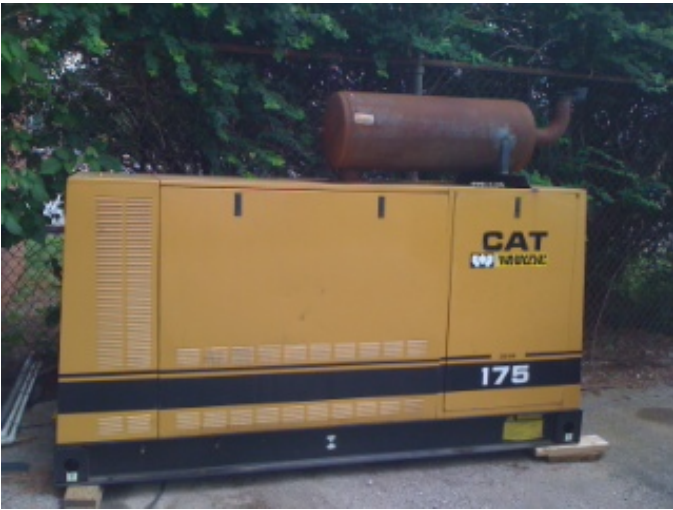
Cat diesel Generator
