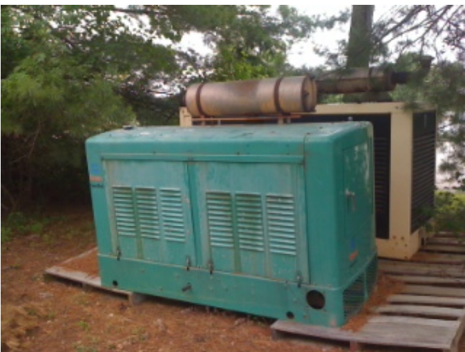
Natural gas powered generator
