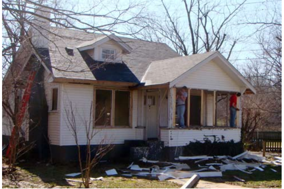
WKU's Campus Chapter of Habitat for Humanity deconstructs a house on Normal Drive
